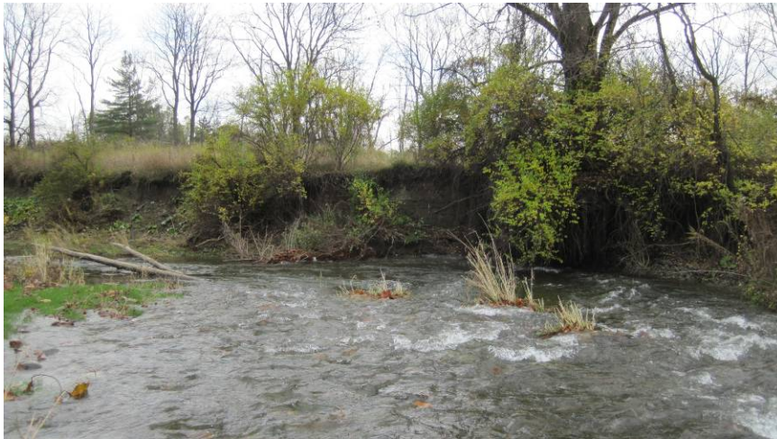
Photo 4: Eroding bank segment in a high bluff.
