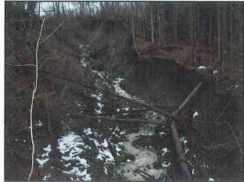
Hedgerow stream channel erosion.
