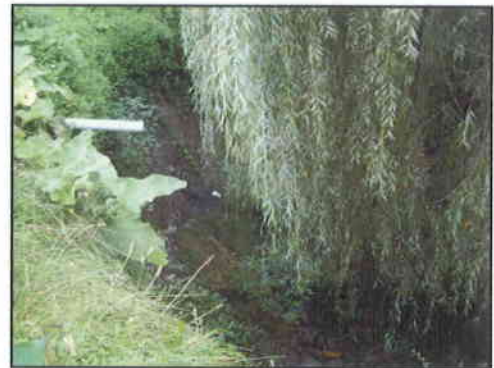
Channel erosion downgradient of Ludlowville Road Culvert 12.
